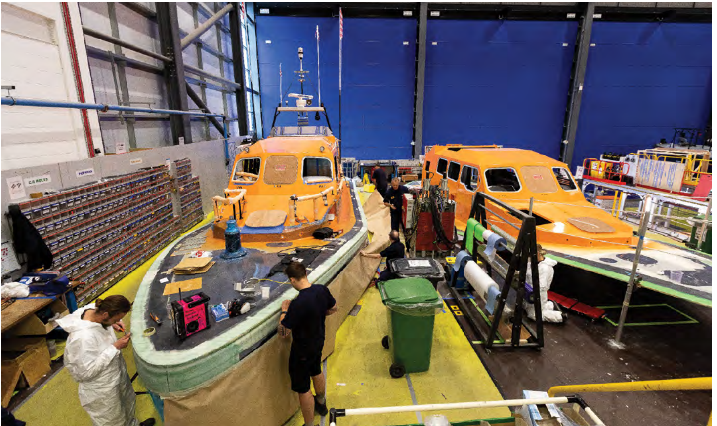
Climate change is rapidly altering the operational context for SAR organisations, requiring a new approach to rescue platform design and construction. For example, these Shannon-class rescue vessels under construction for United Kingdom's Royal National Lifeboat Institute have far stronger hulls than previous designs. This enables rescues in rougher seas and provides greater resistance to debris, which is often present in the water after large weather events. Courtesy RNLI / Nathan Williams
